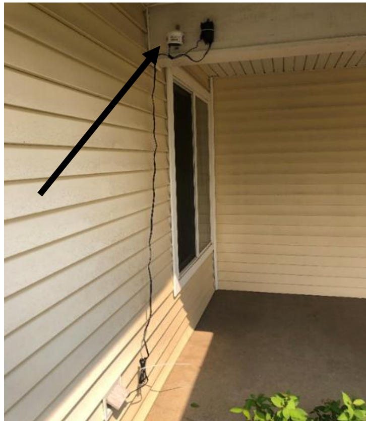
Figure 7. Exterior Sensor Setup @ Facility 2
