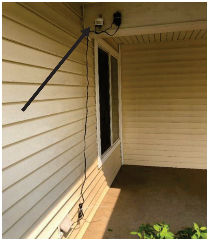
Figure 7. Exterior Sensor Setup @ Facility 2
