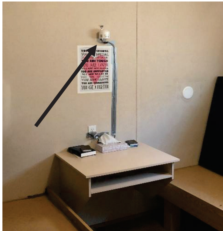
Figure 2. PurpleAir Setup @ Facility 1
