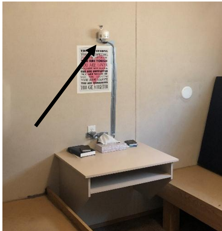
Figure 2. PurpleAir Setup @ Facility 1
