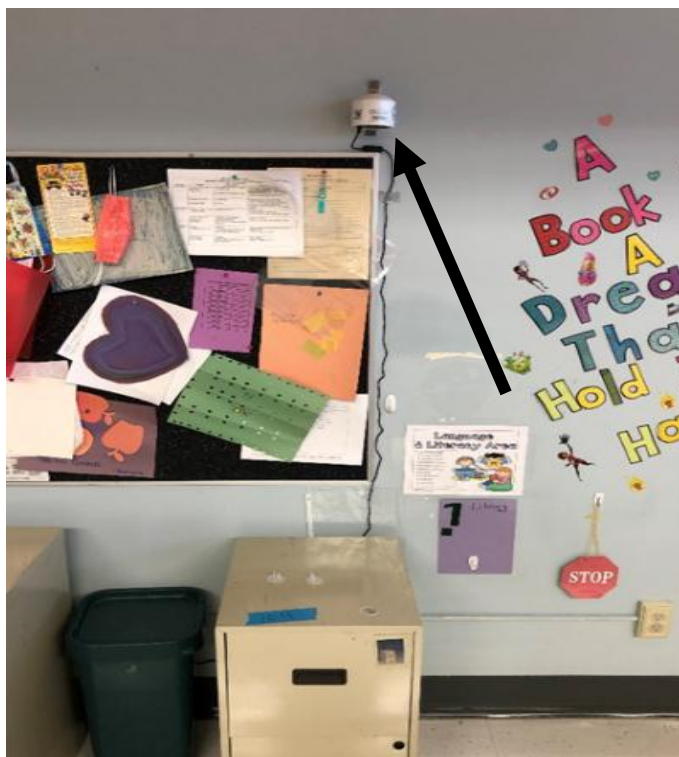
Figure 8. PurpleAir Setup @ Facility 3
