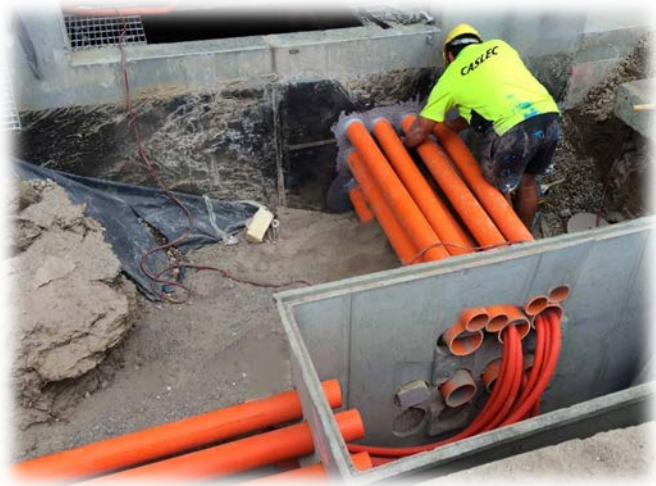
Image credit: Caslec Electrical & Data used is for illustrative purposes only.
