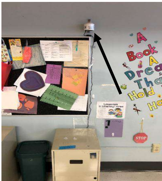
Figure 8. PurpleAir Setup @ Facility 3
