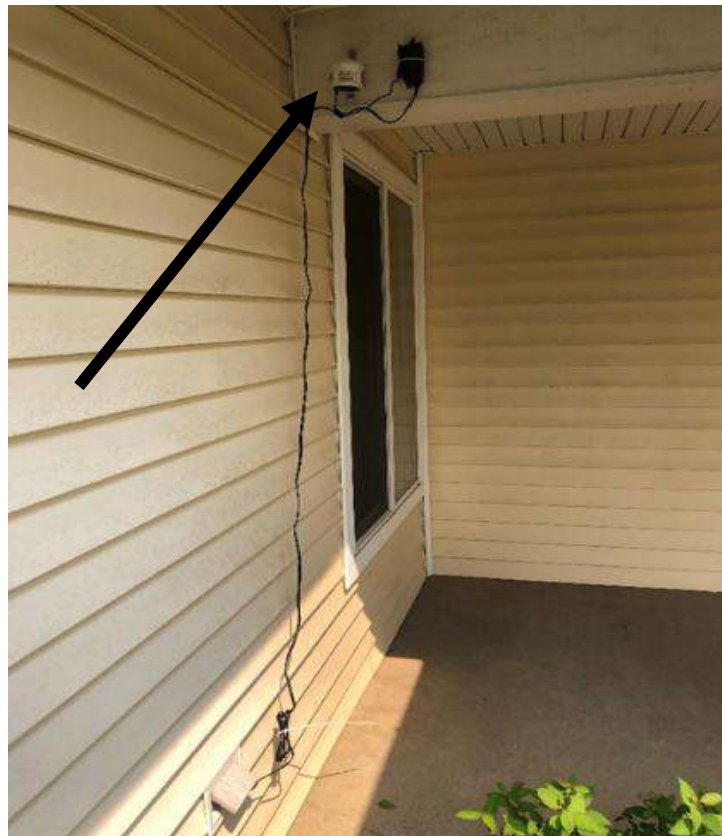
Figure 7. Exterior Sensor Setup @ Facility 2
