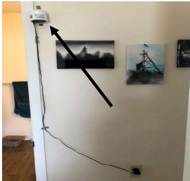
Figure 5. PurpleAir Setup @ Facility 2
